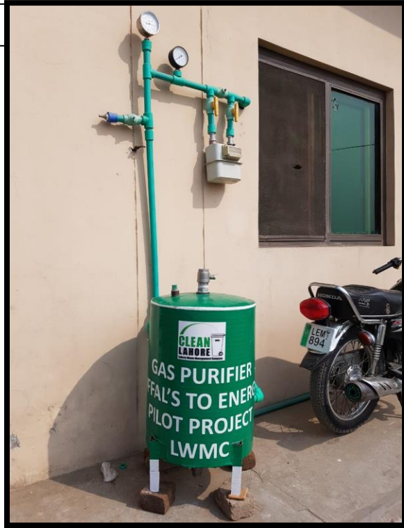
Gas Purification Assembly
