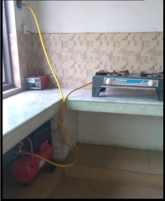
Gas Storage and Stove Assembly
